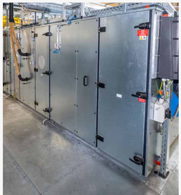
Abb. 8: Air handling unit
